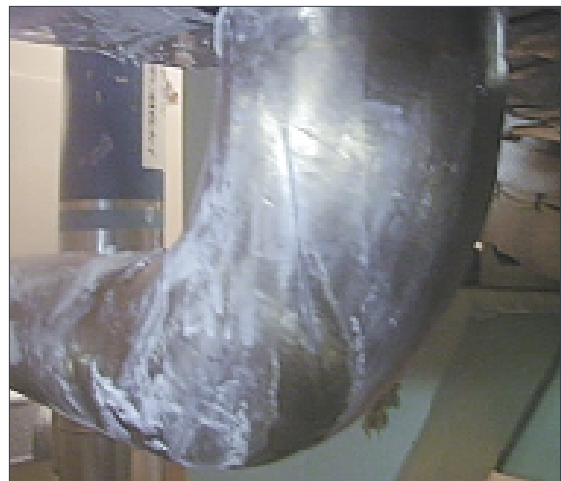
The pipe elbow with the vertical crack that caused the July 12 leak at Tsuruga-2 in Japan (JAPC Photo)
