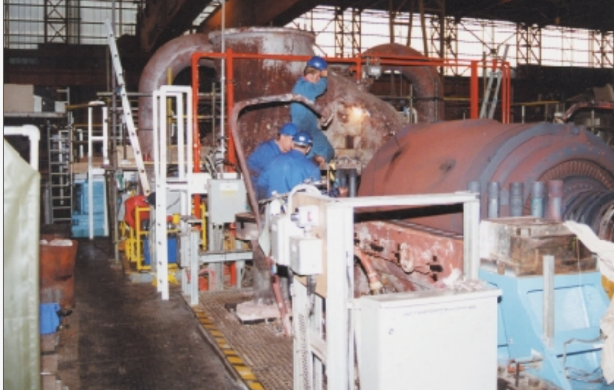
Inspection of a high-pressure turbine module at Heysham-2 station
