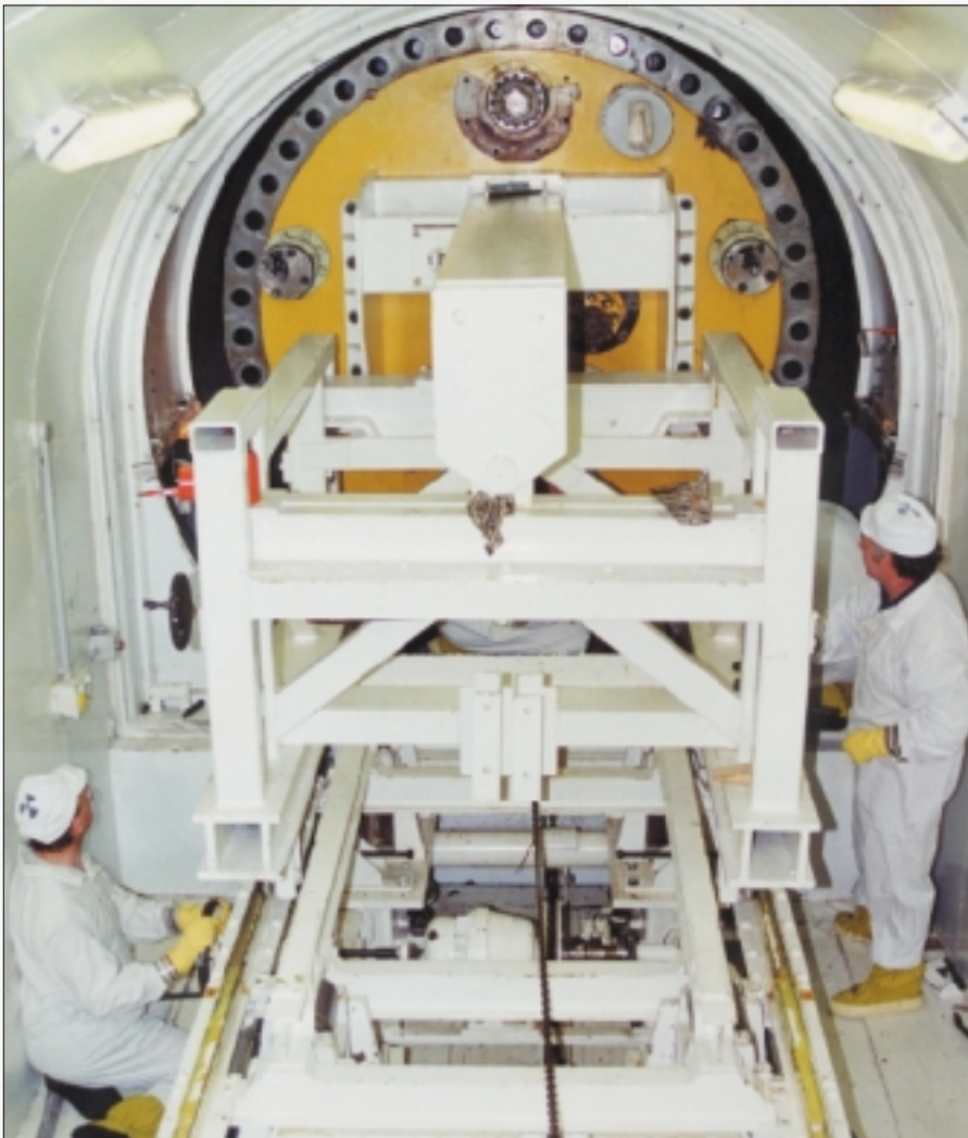
At Heysham-2 station, technicians work down a gas circulator penetration, preparing a gas circulator for removal and subsequent replacement.
