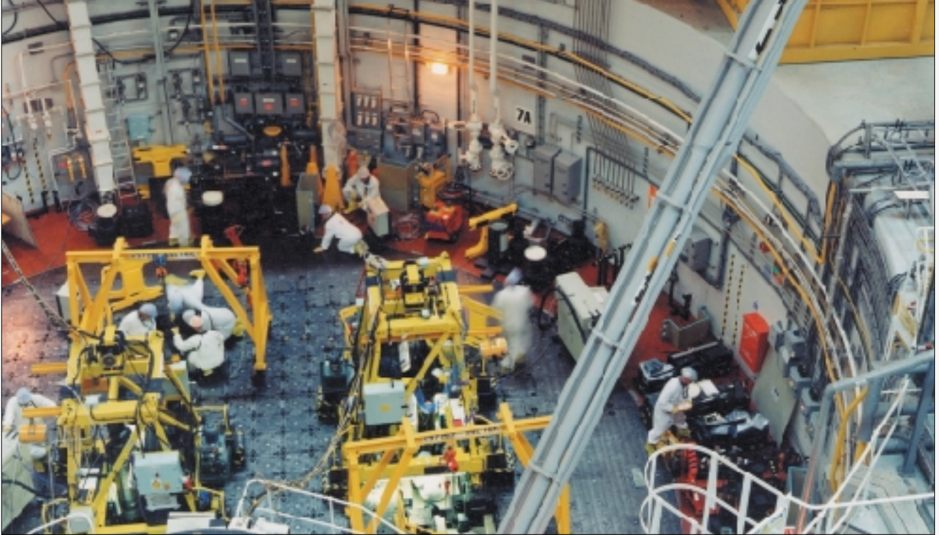
Heysham-2 station's standpipe liner modification project. The work involves modifying the standpipe liner sleeve by drilling a small vent hole about 1 m down each liner tube, using a robotically operated tool.
