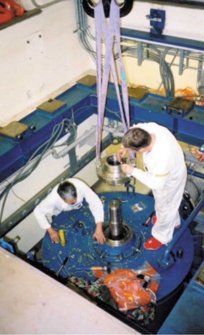
At Leibstadt, mechanics install a coupling on one of the main condensate pumps (NN photo by Dick Kovan)
