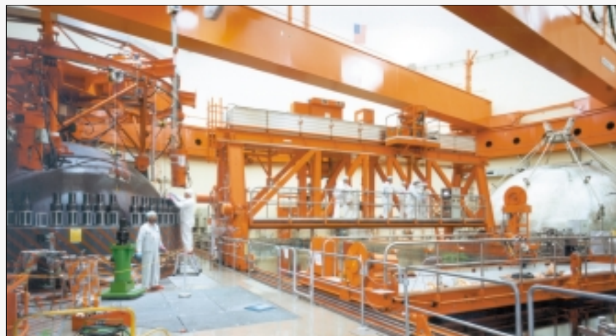
A general view of the refueling floor with the reactor vessel head (left) and drywell head (Source: KKL)
