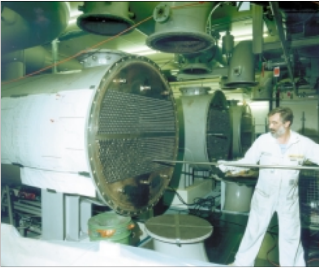
Retubing a heat exchanger in the turbine island closed cooling water system at Leibstadt (Source: KKL)
