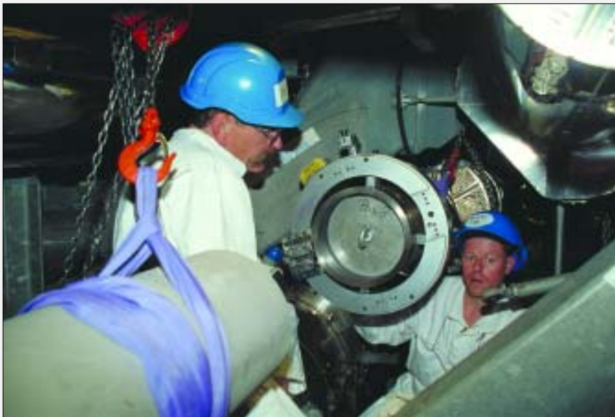
At Forsmark-3, two fitters employed by a contractor prepare a pipe surface for welding of the pipe leading from the reactor vessel behind the fitters. (Photo: Odd Hedberg/Forsmark)
