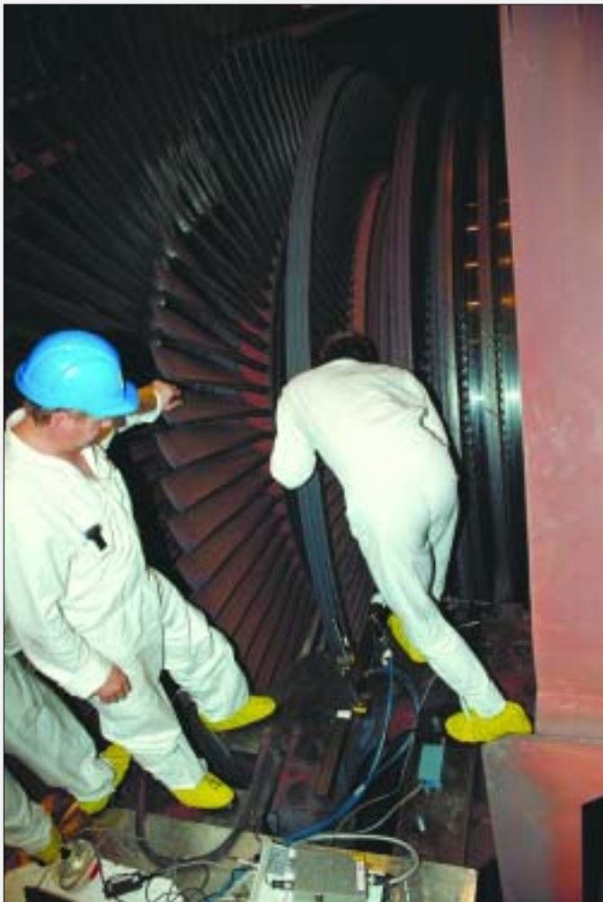
Checking the number two low-pressure turbine rotor for signs of cracking at Forsmark-3 (Photo: Odd Hedberg/Forsmark)
