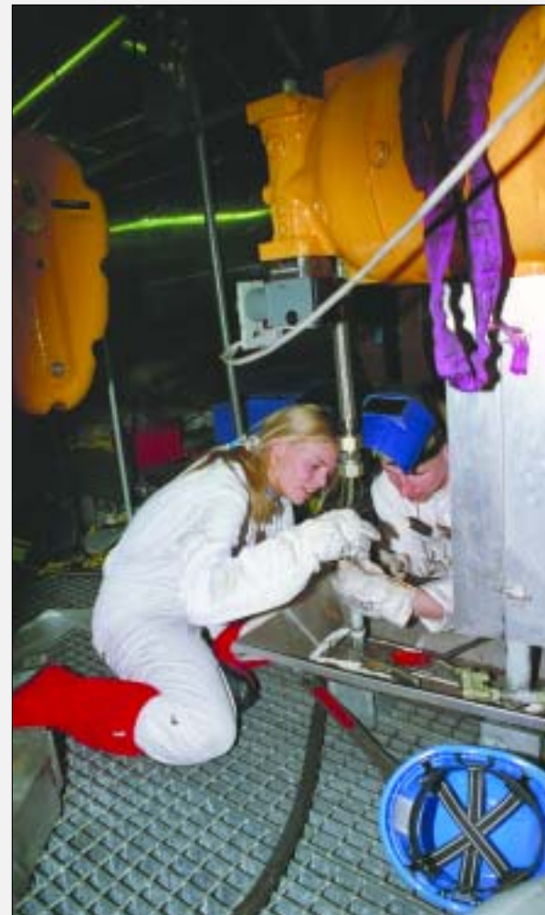
Welders Maja Bjork and Stefan Hellstrom at Forsmark-3 fitting a new valve flange to hydraulic pipe to one of the valve servos. (Photo: Odd Hedberg/Forsmark)
