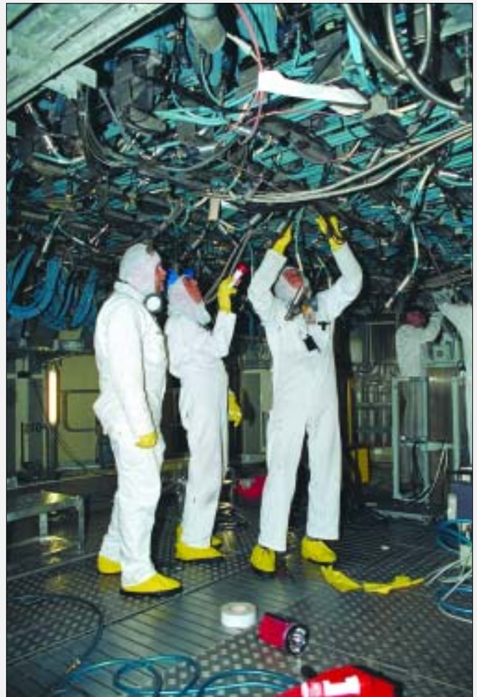
Refitting cabling to one of the control rod actuator motors at Forsmark-3 (Photo: Odd Hedberg/Forsmark)
