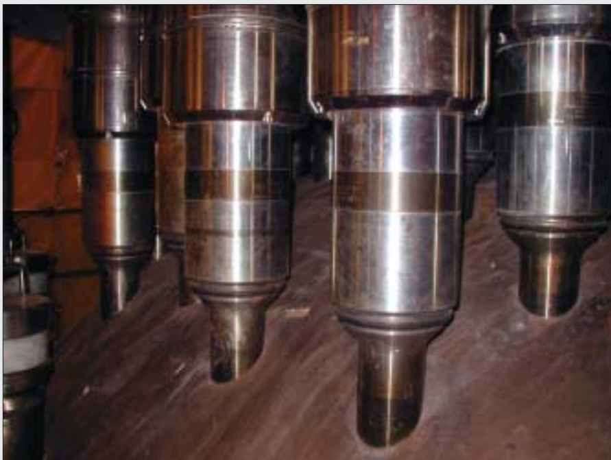
The Calvert Cliffs-2 reactor vessel head was inspected using bare metal visual inspection and ultrasonic testing as required by the Nuclear Regulatory Commission. Inspection results indicated the head to be in "excellent condition," according to Constellation.
