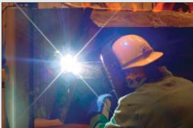
Contract welder Errol Corbin, one of dozens of welders working on the project, practices welding techniques on a girth weld mock-up.
