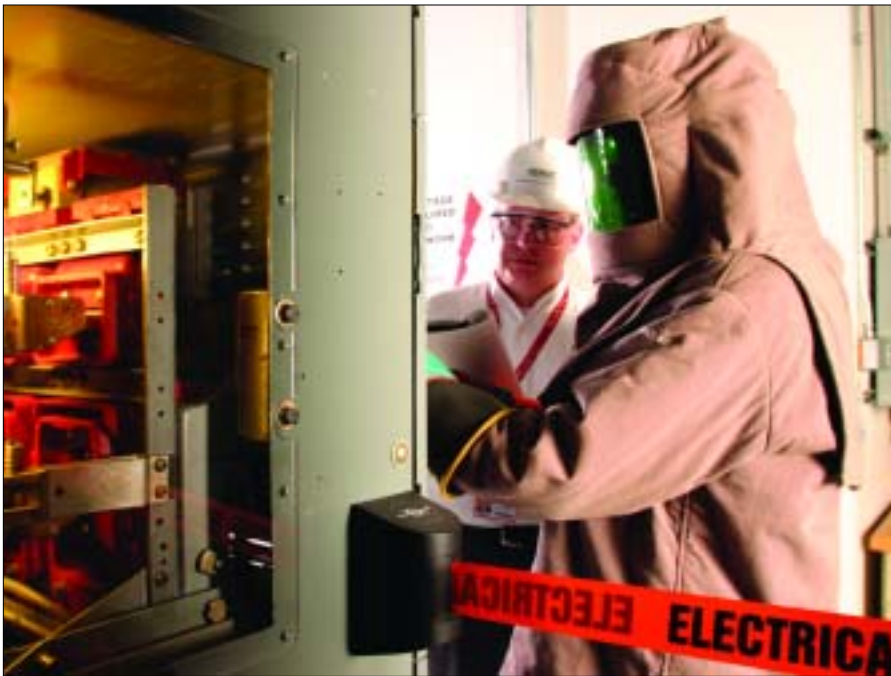
Electrician Jim Palumbo works in full protective gear to rack out a 480-kV circuit breaker on the Perry training simulator flow loop as Mark Monk, lead electrical instructor, observes.
