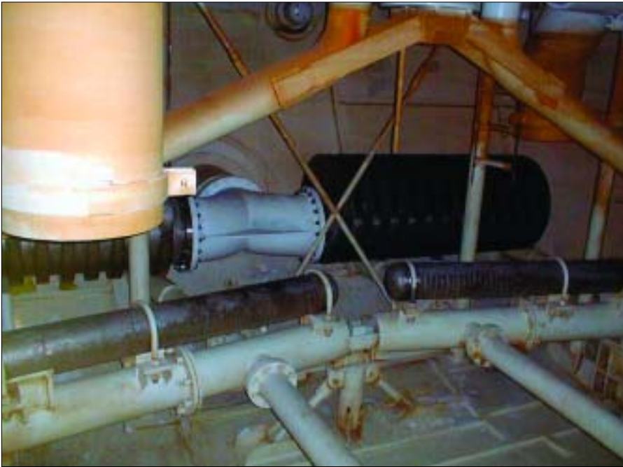
Fig. 1: Photograph of a pair of “stacked disk”-type ECCS suction strainers in the torus of a U.S. BWR Mark I, installed in response to Bulletin 96-03. At Mark I and Mark II BWR units, replacement strainers were cylindrical so as to get them into the wet wells, which have small circular entrance hatches. At PWR units, with much larger equipment hatches, the strainers can be both larger and possibly box-shaped, as opposed to cylindrical. (Photo courtesy of Performance Contracting, Inc.)
