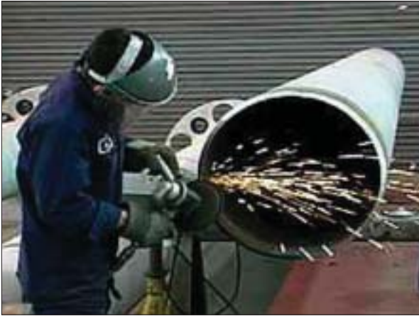
Maintenance worker Jeff Youngblood tests a grinding wheel on a piping segment at the Palo Verde nuclear power plant. (Source: Michael D'Amato/Palo Verde)
