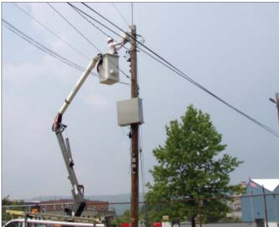
Installation job: Charles Burpoe, senior nuclear environmental monitoring technician at Indian Point, installs a new radiation detector miles away from the plant. (Photo: Eric Weber/Indian Point)
