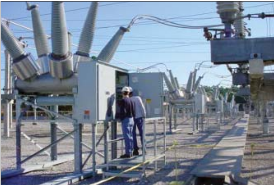
Relay technicians look at new Mitsubishi 230-kV circuit breakers that are being installed in the Surry switchyard to enhance reliability.
