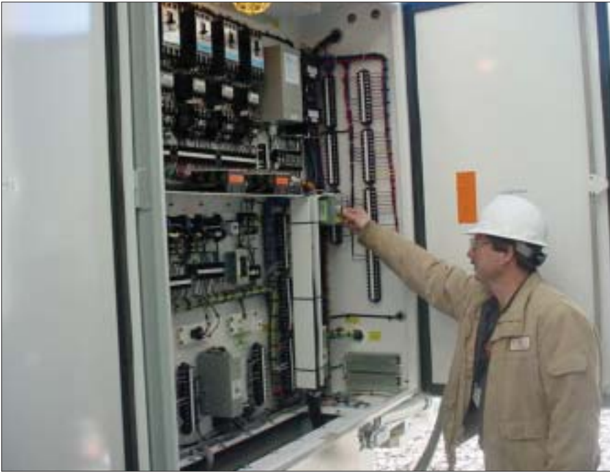
Tim Marshall, senior system protection technician at Surry, checks the fan and cooling controls on one of the new transformers.
