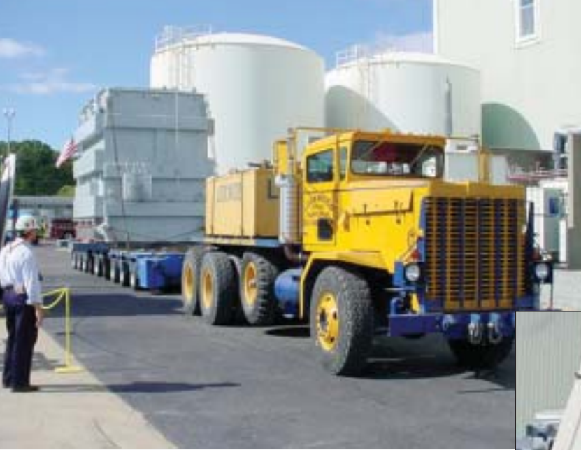
Left: Lockwood Brothers, the load hauler, transports one of the transformers into the Surry station.
