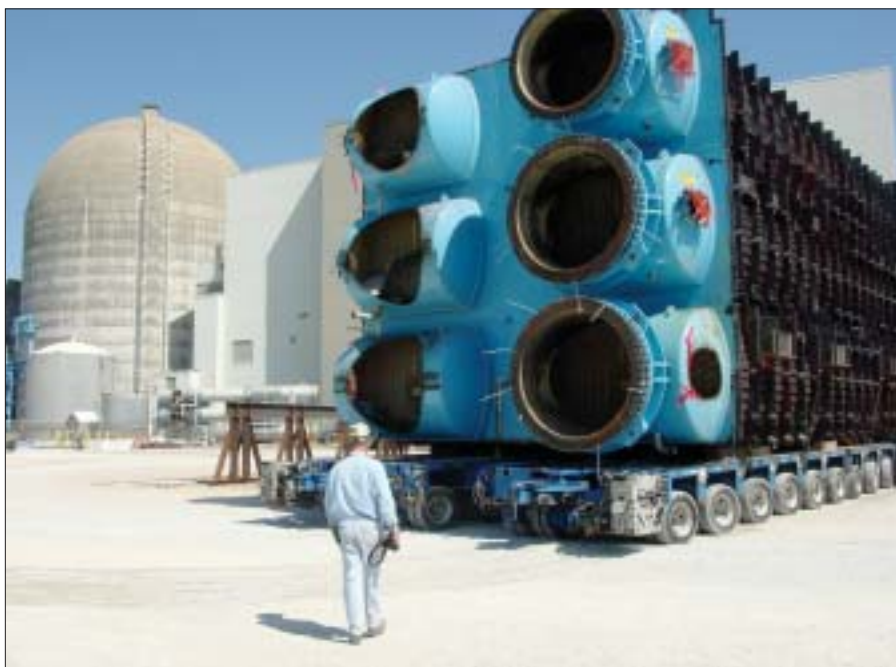
Some of the old condenser tube bundles removed from the turbine building during Callaway's refueling outage in spring 2004.
