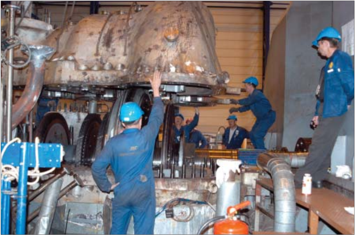
Russian subcontractors overhauling one of the turbines during a 2004 outage at Loviisa (Photo: Seija Niinimäki)
