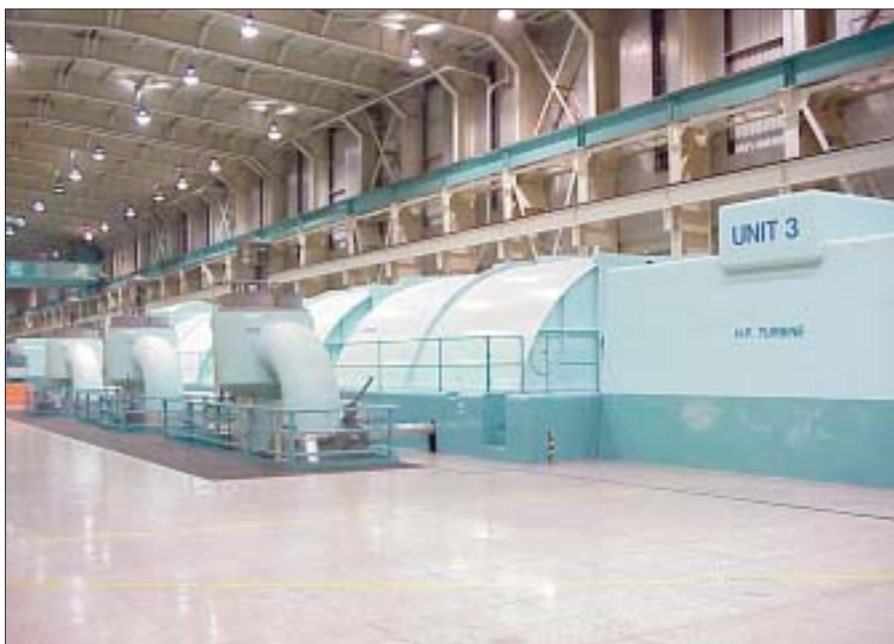
Oconee upgraded to a digital control system for its turbine machinery.
