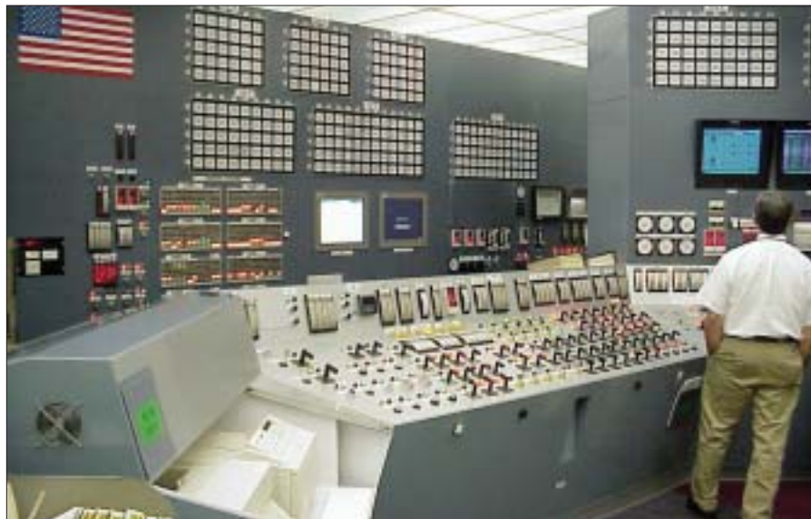
A newly digitized control room at Duke Power's Oconee nuclear power plant replaced dated analog hard-panel interfaces. (Photos: Marlon Dempsey/Oconee)
