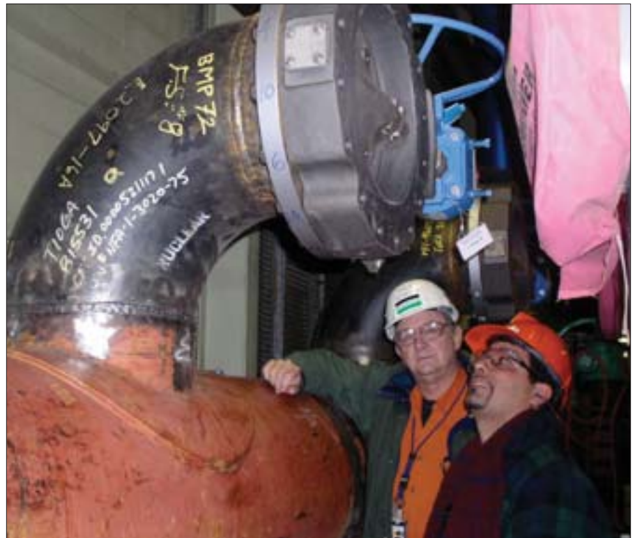
Pickering-1 modifications team leader John Ieraci (right) and Dale Renouf, of contractor Black & McDonald, examine work in progress on the cooling water system. (Photo: Ontario Power Generation)
