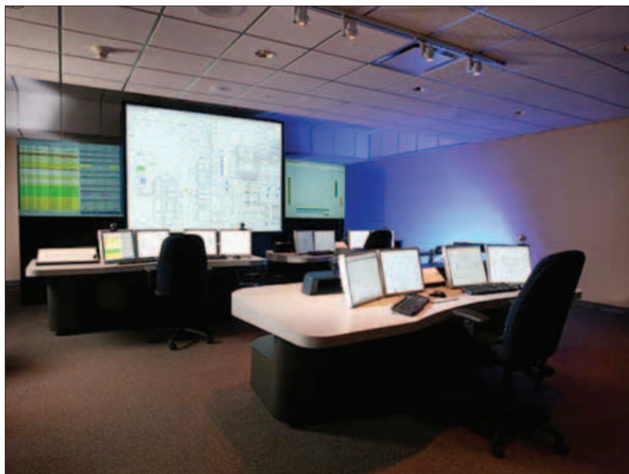
What a new digital I&C control room for Westinghouse's API000 will look like, as shown in a presentation at the NRC briefing
