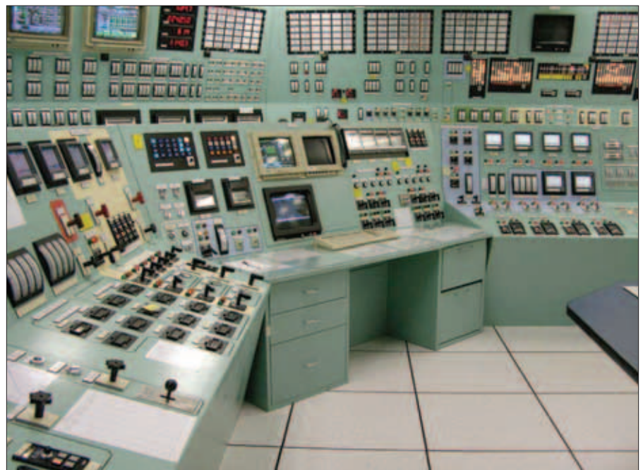
The control panel in a current nuclear power plant
