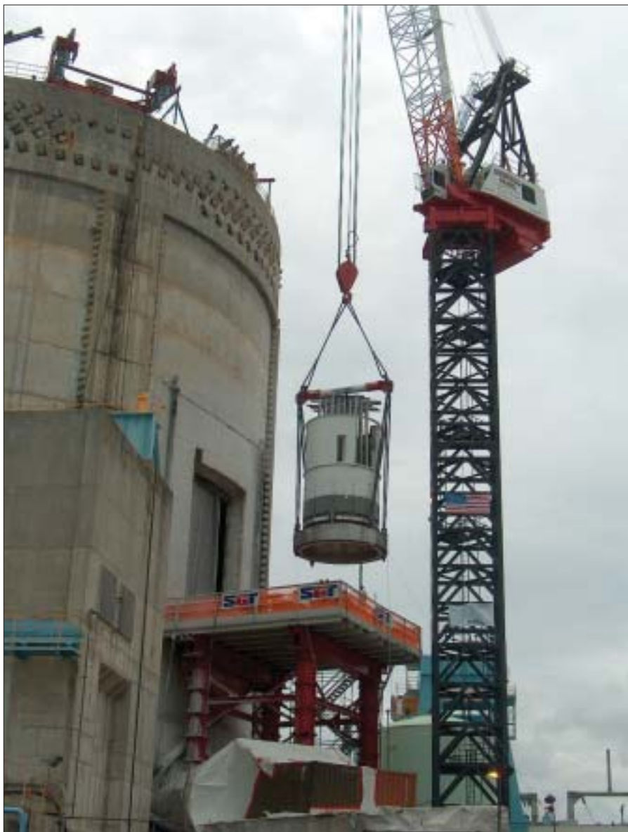
The new reactor head is suspended from the tower crane before being placed on the service platform.
