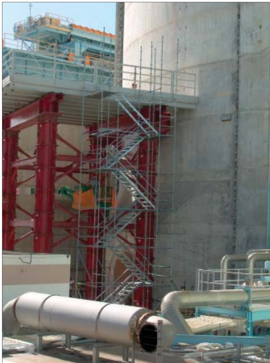
A service platform was constructed next to Turkey Point-3's containment building. Faint orange markings on the concrete wall indicate the "cut line" where an opening would later be created in order to move reactor heads in and out of containment. (Photos: FPL)
