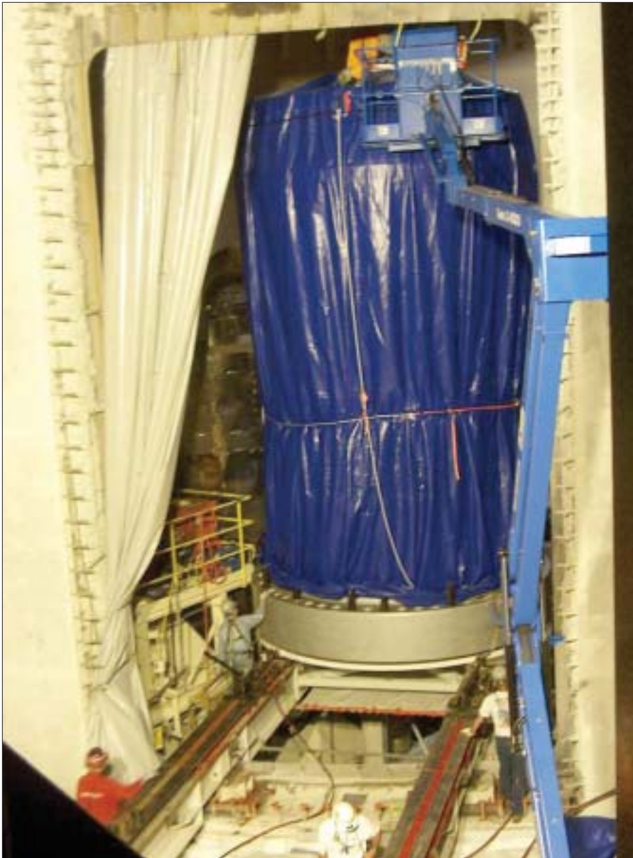
The unit's old reactor head was wrapped in a blue cover before leaving containment through the construction opening.
