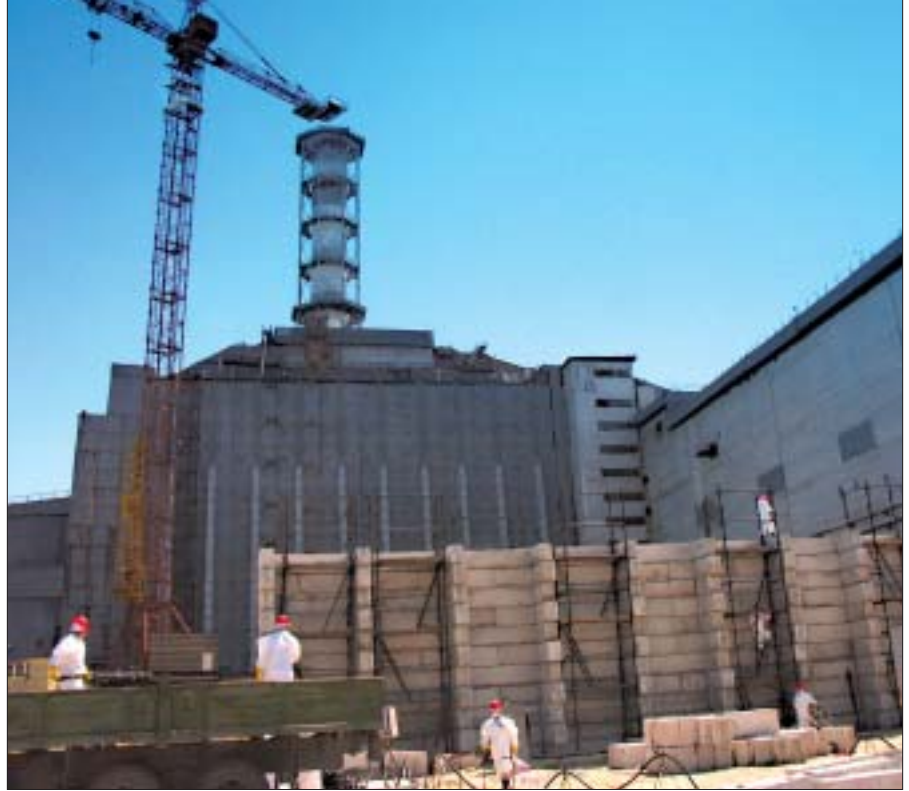
Workers do preparation work for the stabilization of the western wall. (Photo: Insight )
