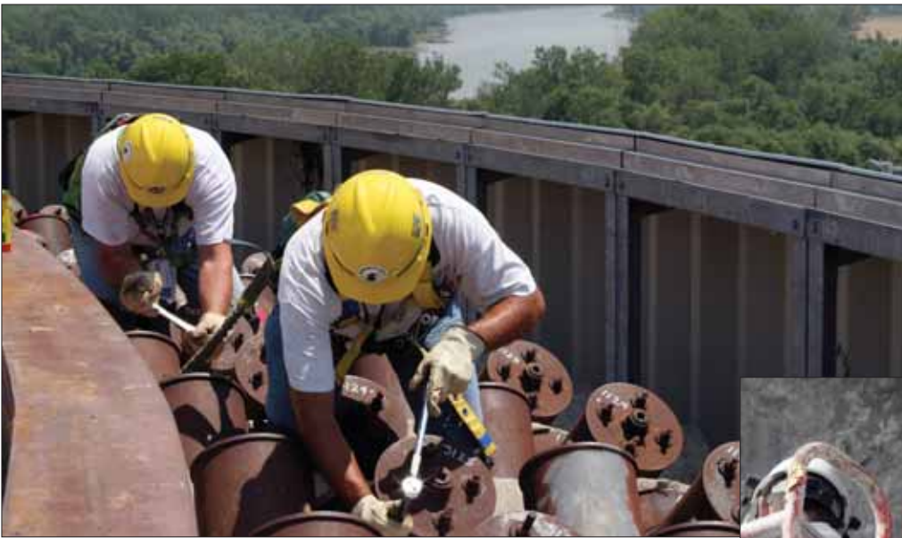
Left: Workers loosen tendons on the top of Fort Calhoun's containment building before their removal so that an opening can be created in the side of the containment building. The tendons are used as just one measure to keep the containment building tight and secure, similar to twine tied around a package.
