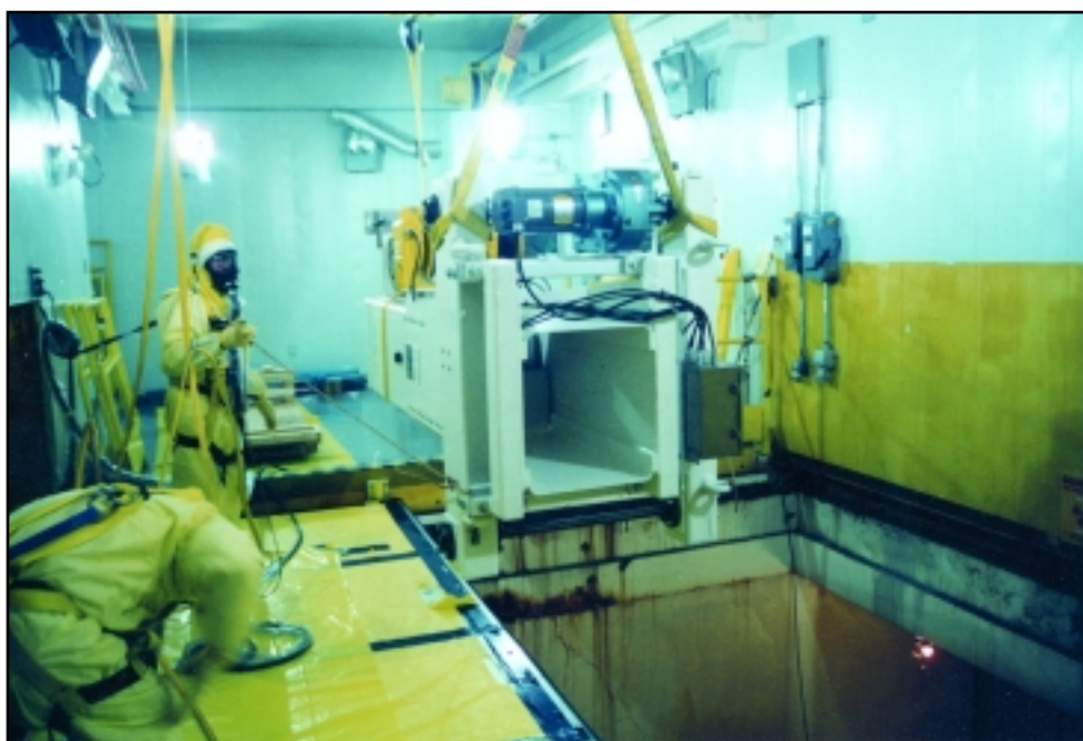
Installing the new crane in the PMC. Workers are tied off for safety.
