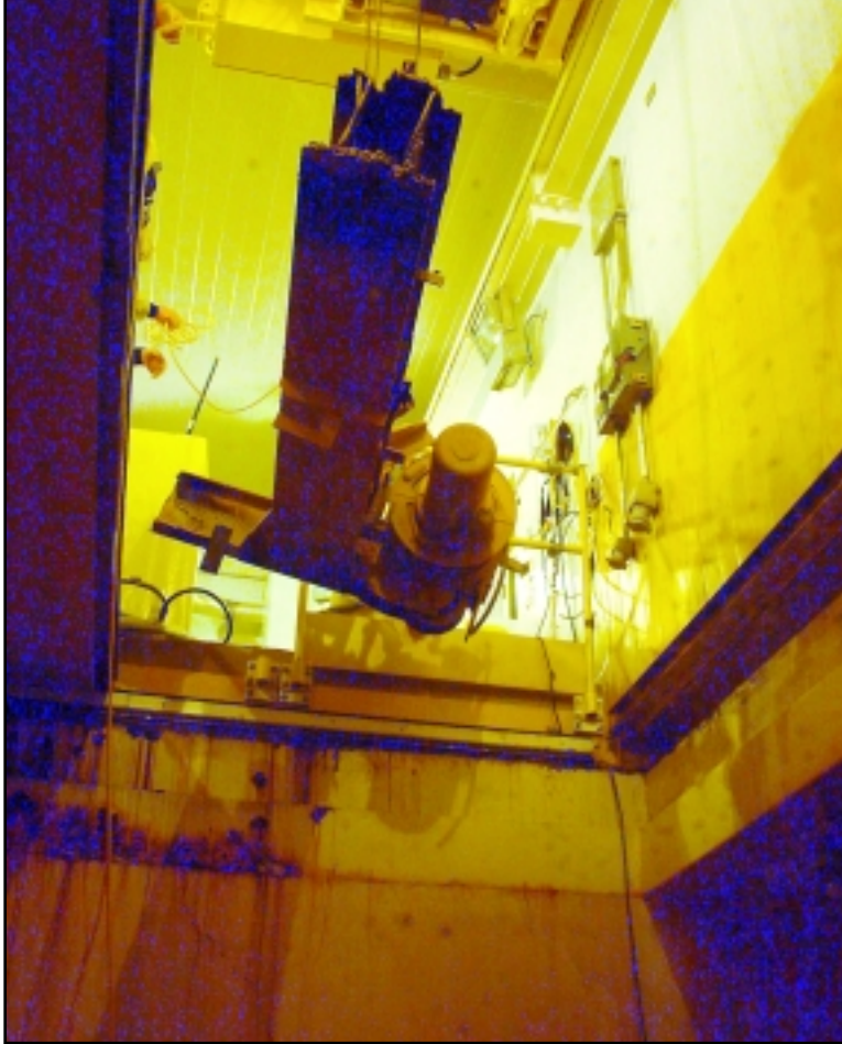
Following size-reduction, the crane pieces were lifted out of the crane room for placement in the waste container.
