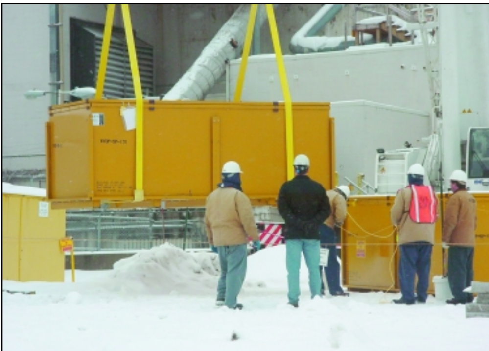
The waste container filled with the size-reduced crane is lowered to the ground for movement to a waste storage area at the WVDP.
